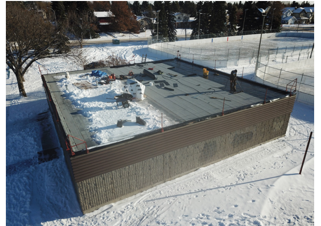
The RCL improved the lighting and roof at Brookside Hall to have a welcoming space available for community-group use.
