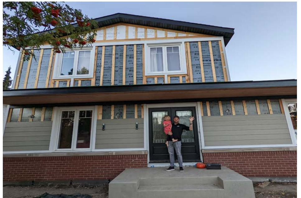
April and her family replaced basement windows, upgraded attic insulation and added rigid foam insulation to the exterior.
